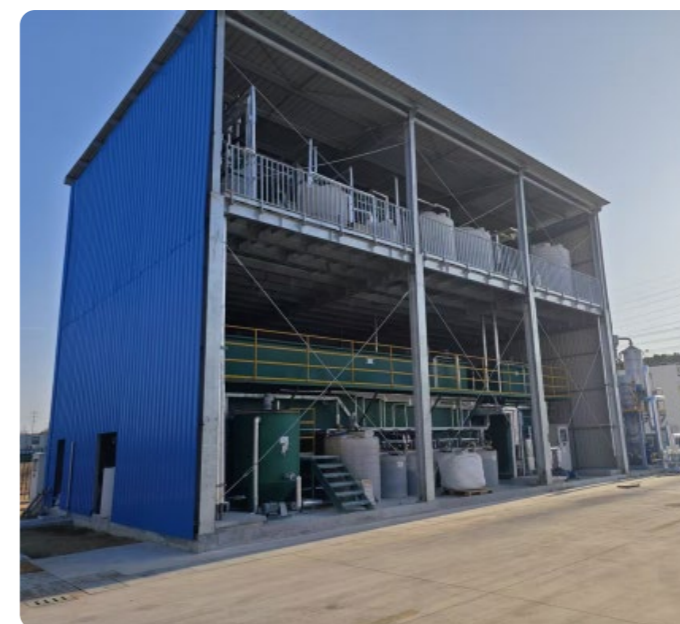
Picture of the wastewater treatment facility at Morimatsu Suzhou Plant
