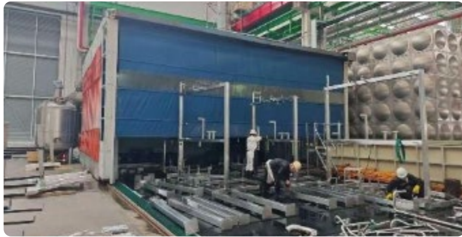
Morimatsu Suzhou Plant Pickling Process Exhaust Ventilation Facilities
